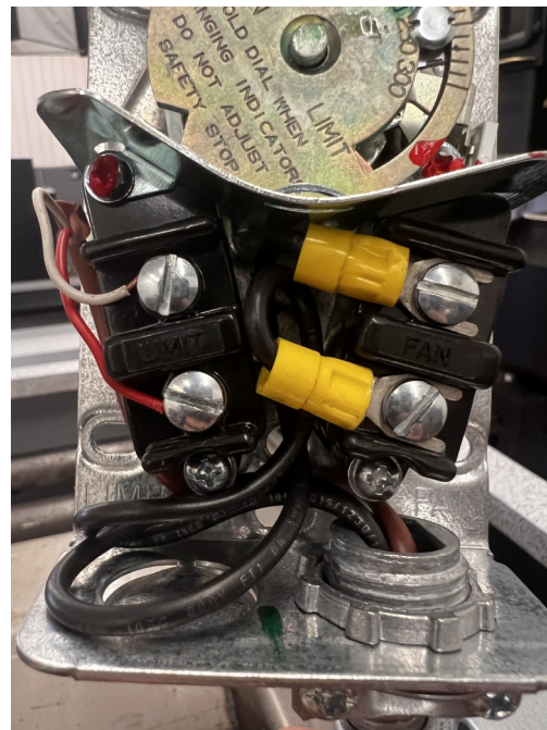
Wiring the fan/limit control
