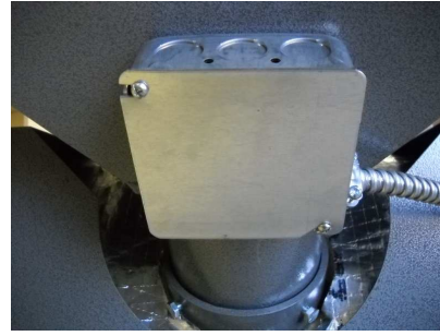
Hopper Temperature Safety Switch: Cover Replaced
